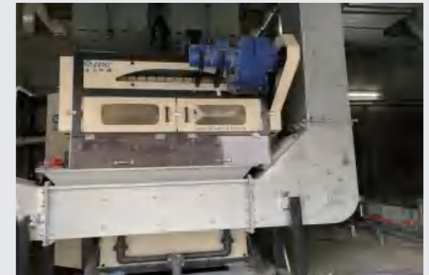
Sludge press roll equipment
