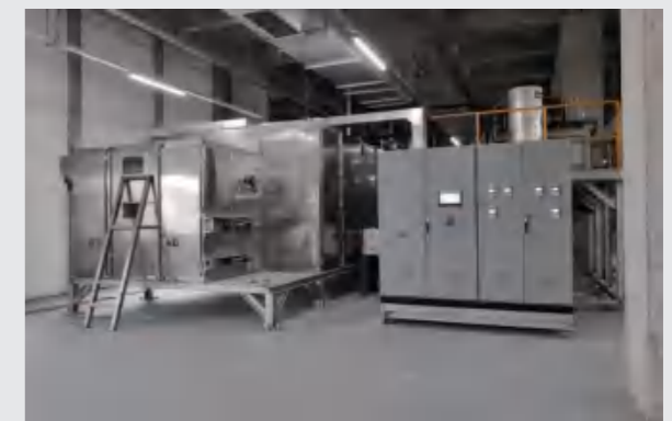
Panel BG copper sludge drying equipment
