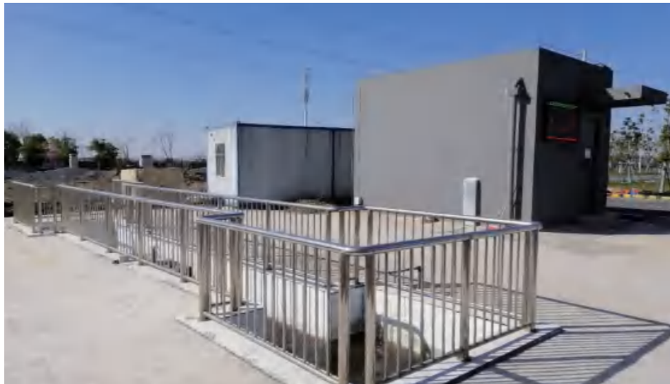
In-line pumping station at the main outfall of the effluent plant
